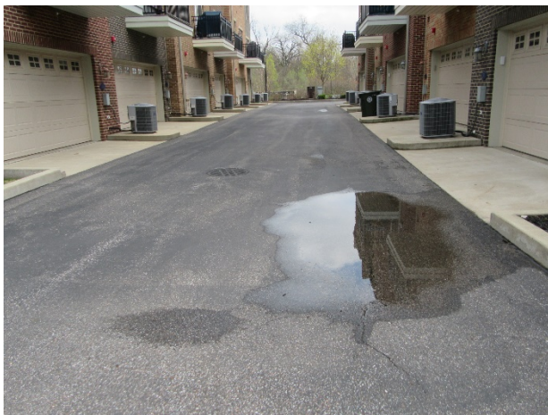
Overview of access drive between Buildings 4 and 5 (note water accumulation)
