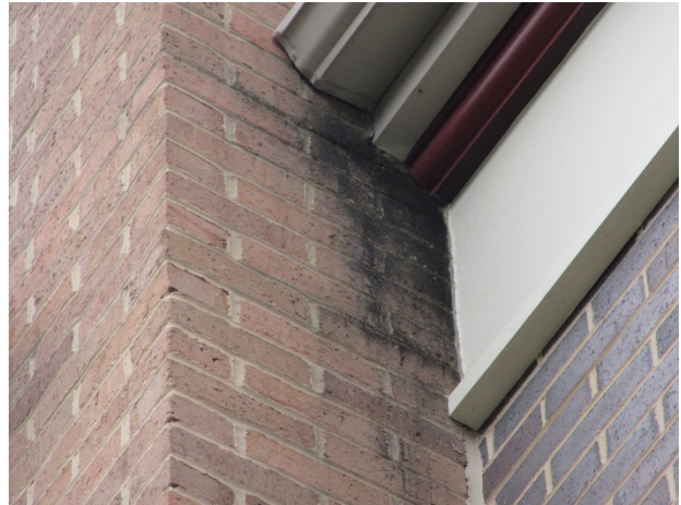
Evidence of overflow at front of Unit 23
