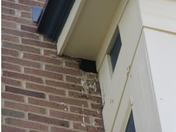
Gap at Unit 19 (noted bird infiltration)
