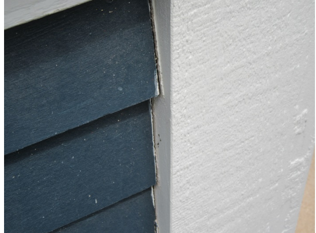
Lack of sealant at Unit 24
