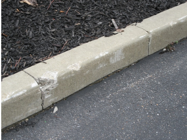
Curb damage near Unit 41
