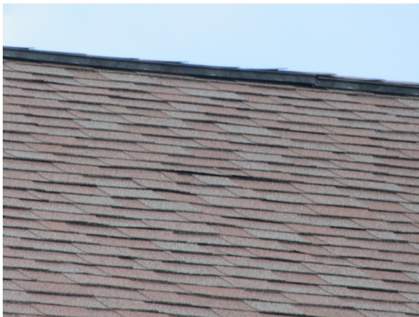
Sheathing deflection at Unit 24
