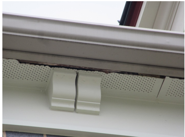
Soffit damage at Unit 98
