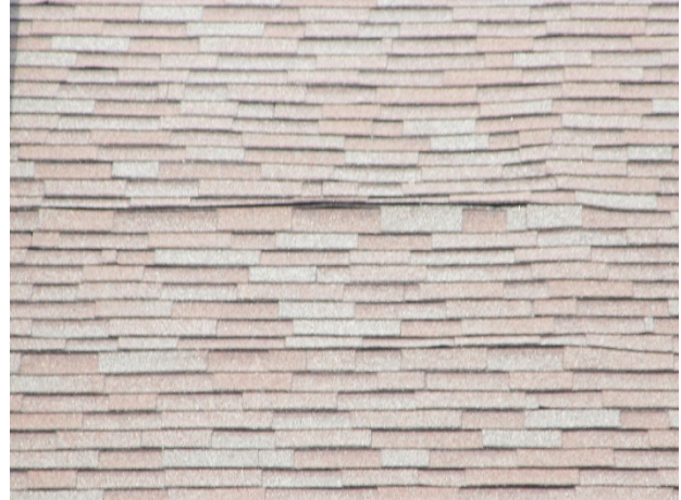
Sheathing deflection at Unit 97
