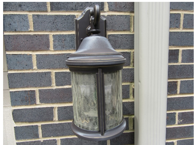
Finish deterioration at Unit 61
