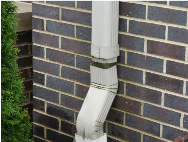
Disconnected downspout section at front of Unit 16
