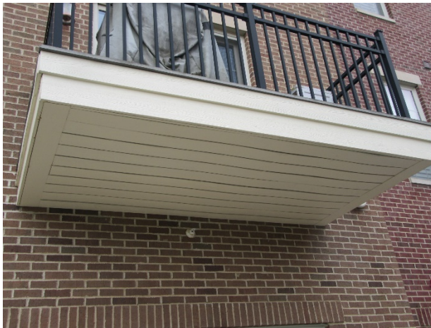
Typical deflected soffit
