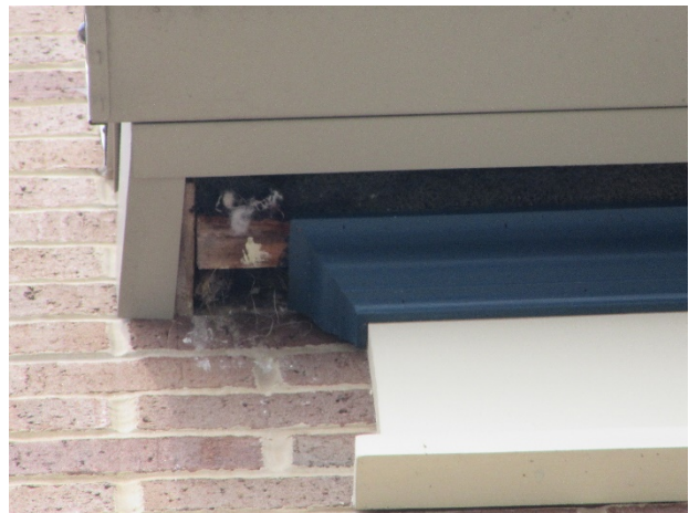
Missing soffit at Unit 54
