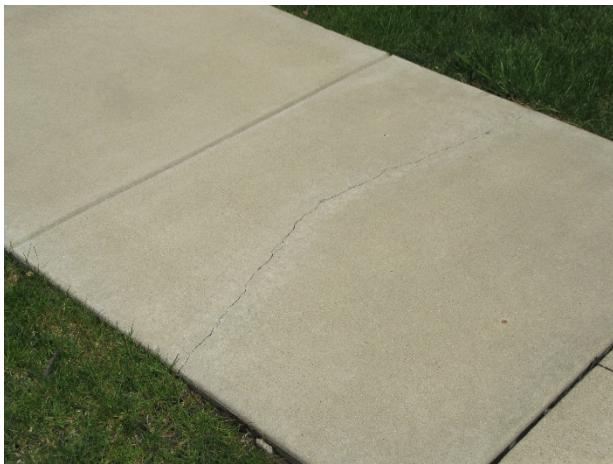
Crack at Unit 33
