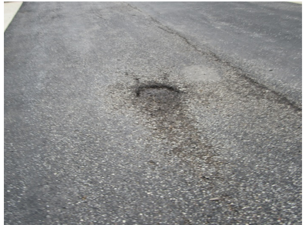
Localized deterioration near Unit 32
