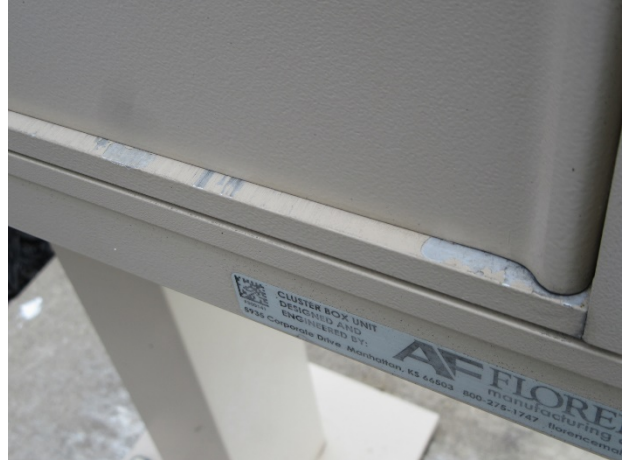
Minor finish deterioration near Unit 55
