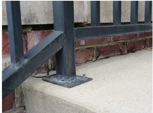
Spalled masonry and deterioration at Unit 24
