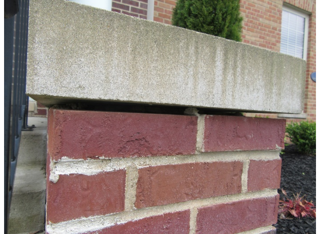
Missing mortar at Unit 12
