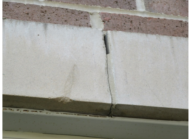
Mortar crack at Unit 19
