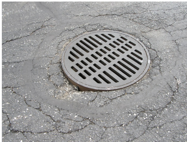
Settlement near Unit 11
