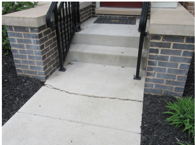
Crack at Unit 92
