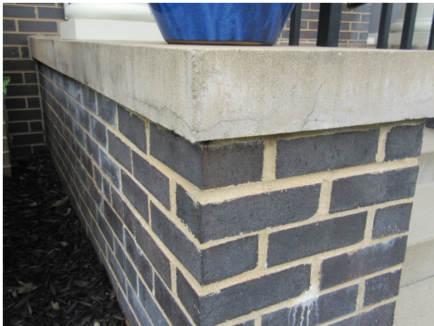
Capstone cracks and efflorescence at Unit 23
