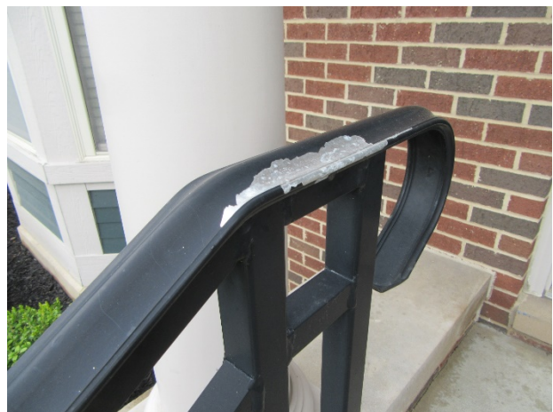
Finish deterioration at Unit 17
