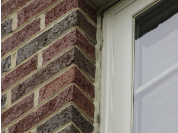
Adhesive sealant failure at front of Unit 17
