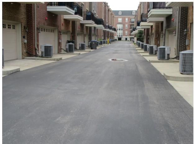
Overview of access drive between Buildings 6 through 9 (note water accumulation)
