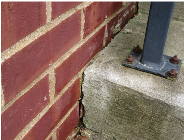
Opportunity for water accumulation between stairs and wing wall masonry (note deterioration)
