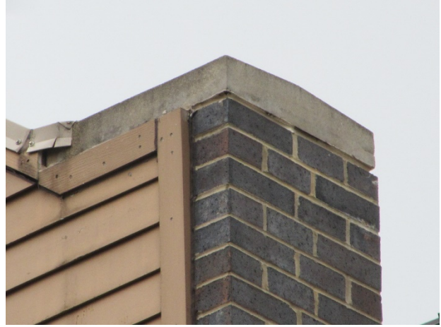
Siding installed offset from parapet wall at Unit 45 (opportunity for water infiltration)
