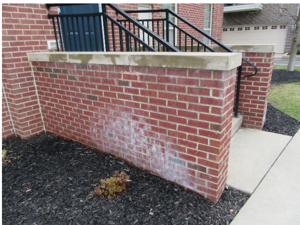
Efflorescence at Unit 46
