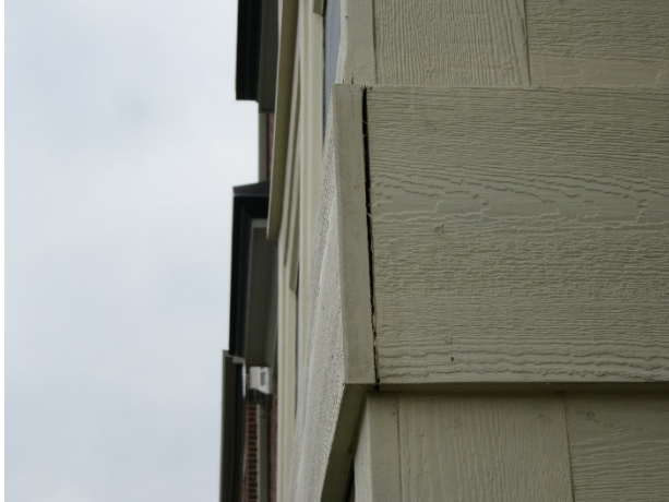
Loose trim at Unit 35
