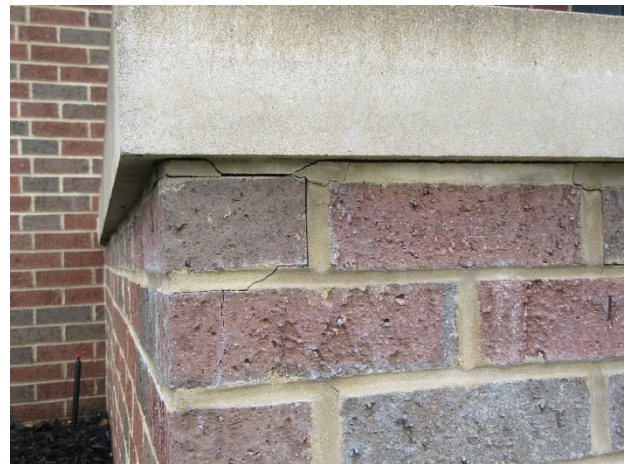
Wing wall mortar cracks at Unit 15 (note undersized capstones)
