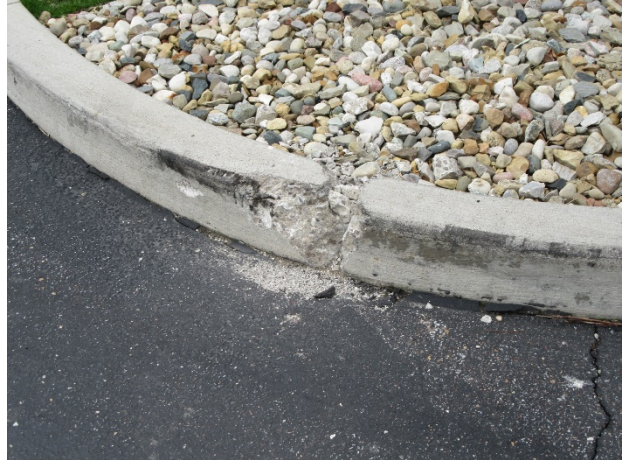
Curb damage near Unit 55
