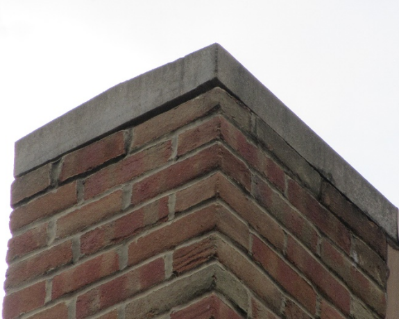
Gap at Unit 33
