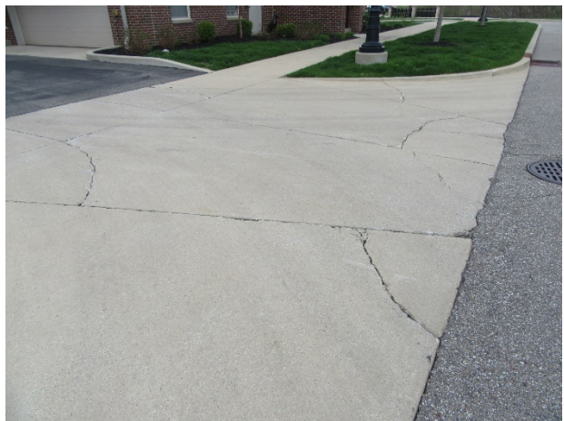
Cracks near Unit 98
