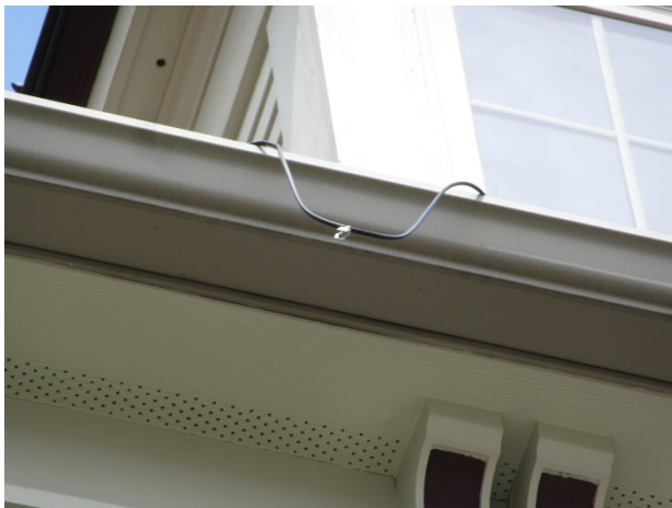
Loose heat tracer at Unit 51
