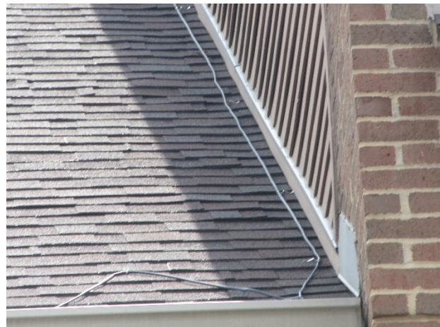
Minor shingle lift at Unit 66
