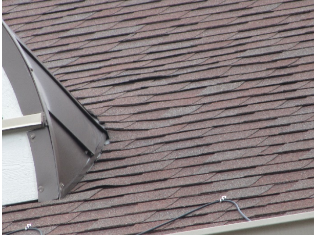
Raised shingles at Unit 53
