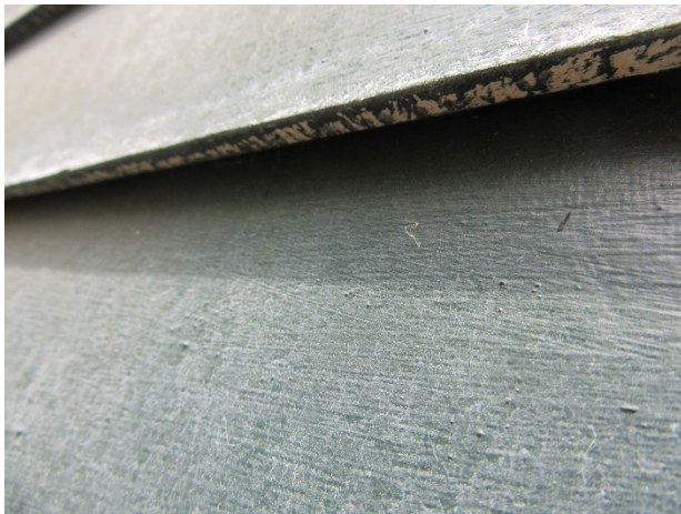
Paint coverage issue at front of Unit 32
