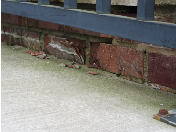
Spalled masonry at Unit 14
