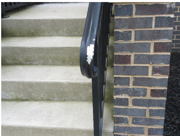
Finish deterioration at Unit 66
