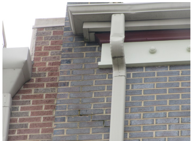
Mortar deterioration likely exacerbated by water runoff at Unit 16
