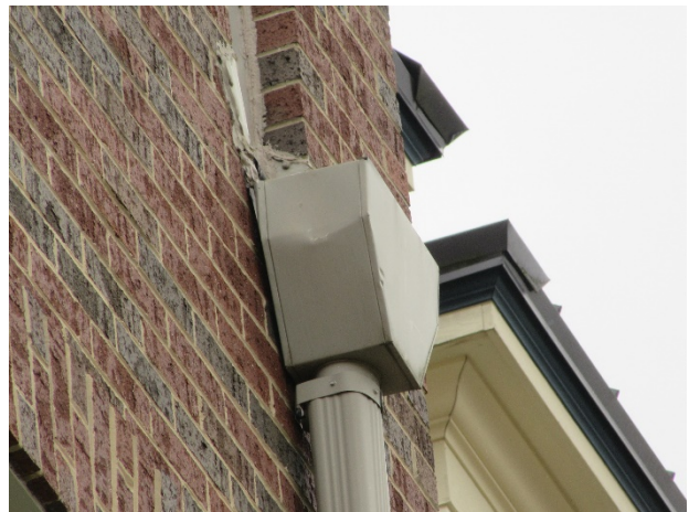
Additional sealants and likely overflow issue at Unit 35
