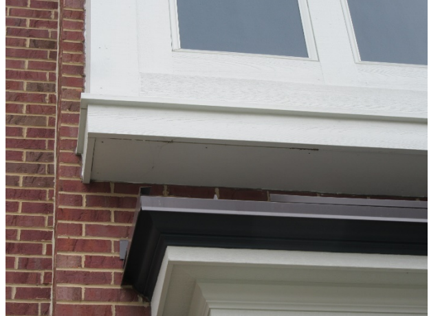
Deterioration and potential water infiltration at Unit 46
