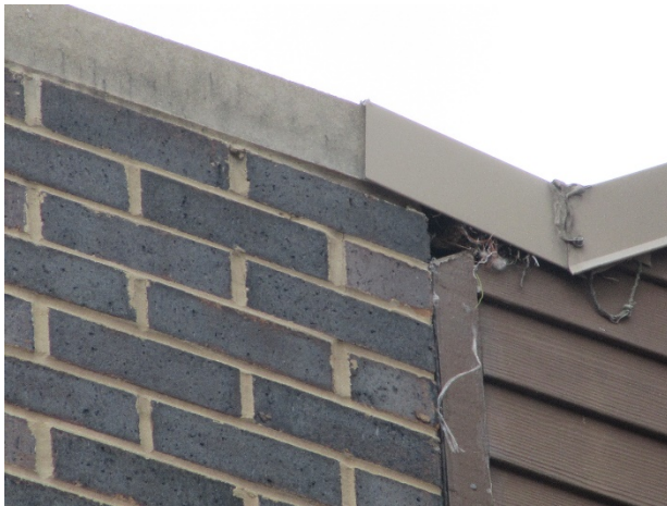
Damage at Unit 86
