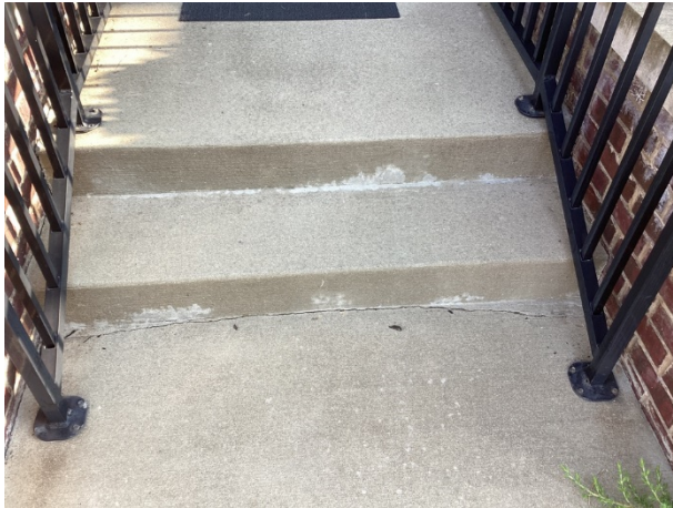
Stair cracks at Unit 87
