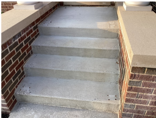
Concrete stairs with spall and removed railing
