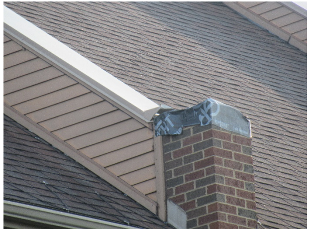
Aluminum wall cap missing – Note: ongoing repairs, we assume installation of cap in near term
