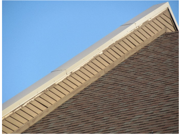
Parapet walls overview with minor finish deterioration
