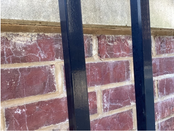
Cracks and scaling masonry at Unit 71
