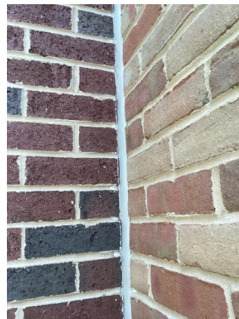
Adhesion failure at Unit 43
