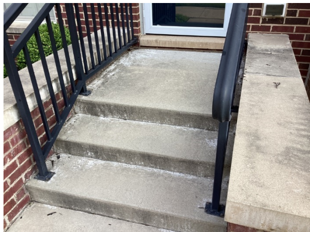
Concrete stairs with staining
