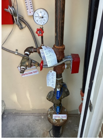
Rusted sprinkler valves
