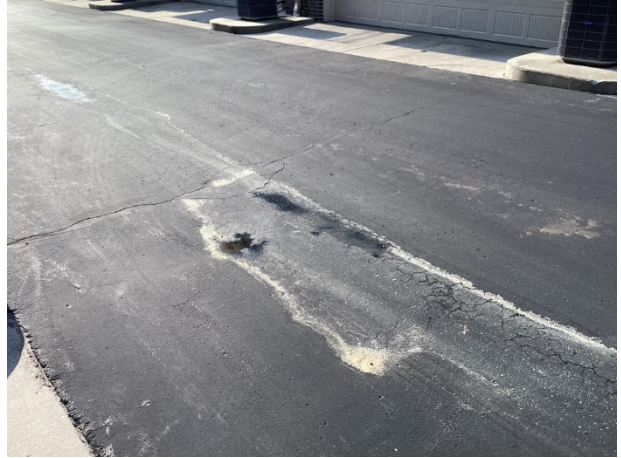
Pavement longitudinal cracks and alligator cracks
