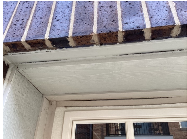
Cohesive failure above garage
