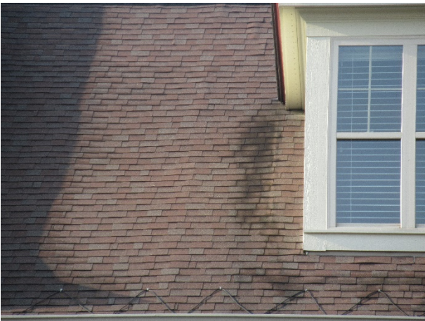
Asphalt shingle roof staining
