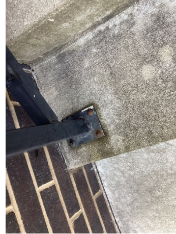
Rusted fasteners at Unit 45
