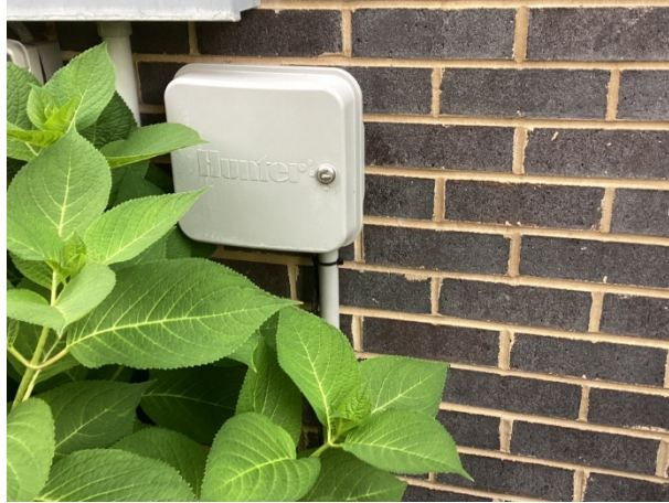
Irrigation system controller
