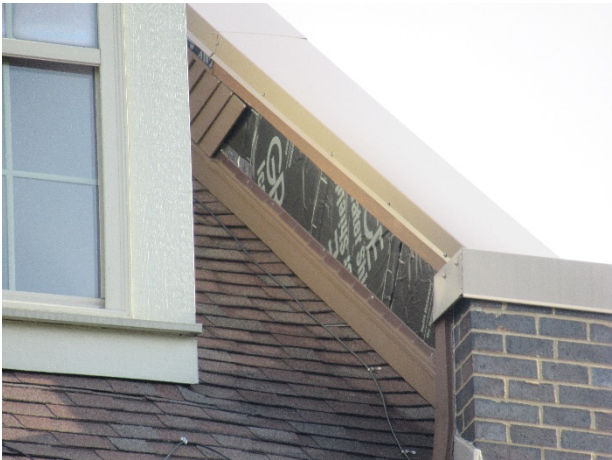
Missing siding at parapet wall – Note: ongoing repairs, we assume installation of siding in near term
