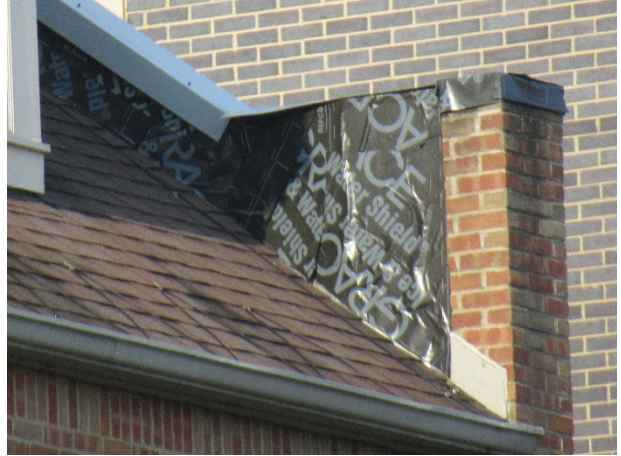
Missing siding at parapet wall – Note: ongoing repairs, we assume installation of siding in near term
