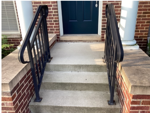
Railing with rusted fasteners
