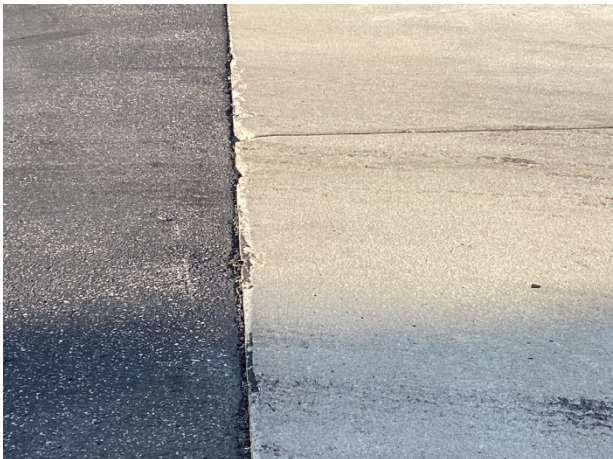
Spall at concrete apron
