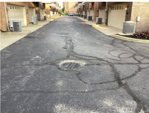
Asphalt pavement street overview with cracks and repairs
