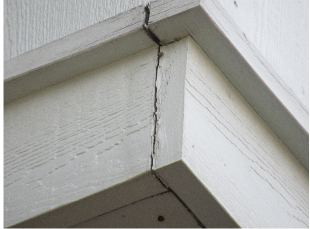
Loose trim boards
