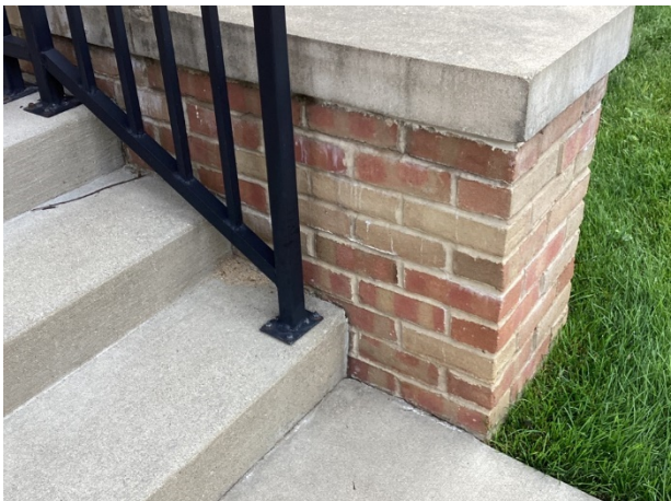
Masonry cracks and missing sealant at wing wall – Note: opportunity for water accumulation between stairs and wing wall masonry
