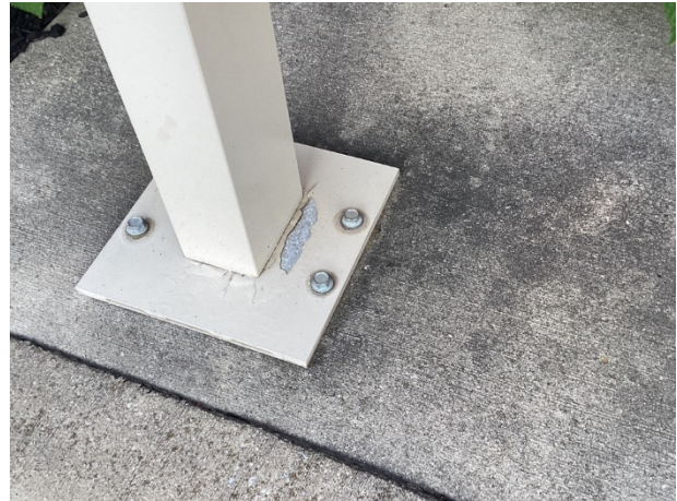
Mailbox station minor finish deterioration
