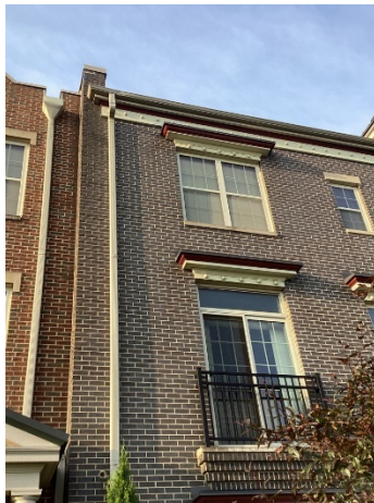
Aluminum gutter and downspout with damaged gutter
