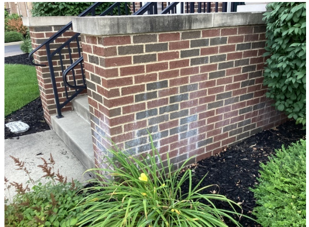
Efflorescence at wing wall
