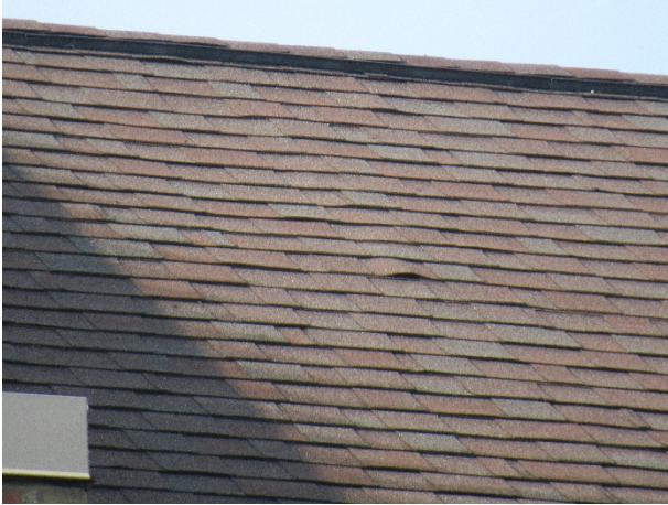
Minor shingle lift
