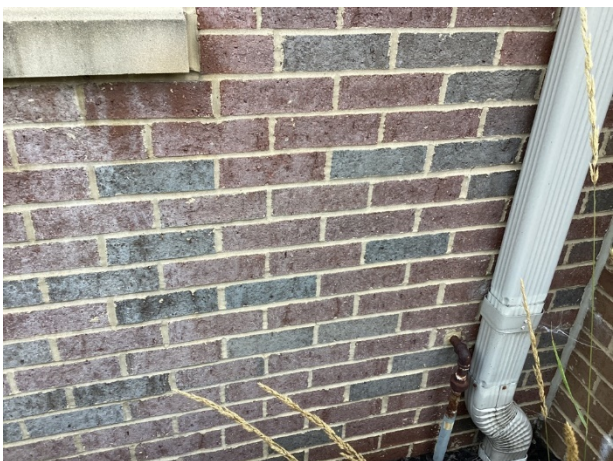
Efflorescence and masonry cracks at Building 2
