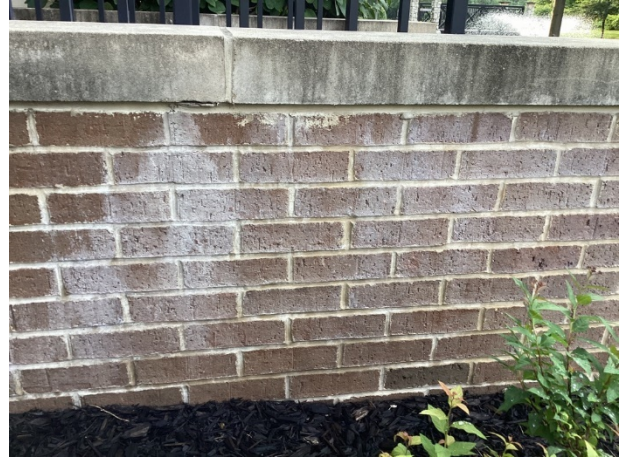
Wing wall efflorescence at Building 2
