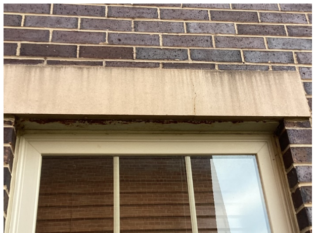
Lintel rust and cast stone crack
