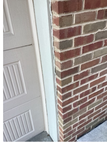
Cohesive failure at Unit 85
