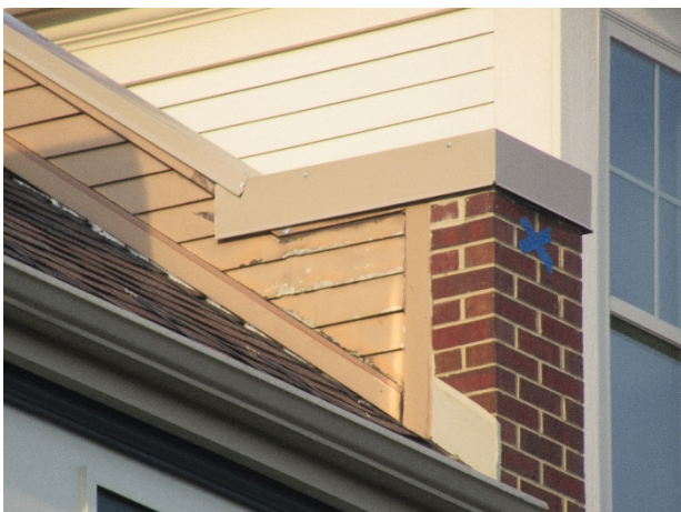
Parapet wall finish deterioration
