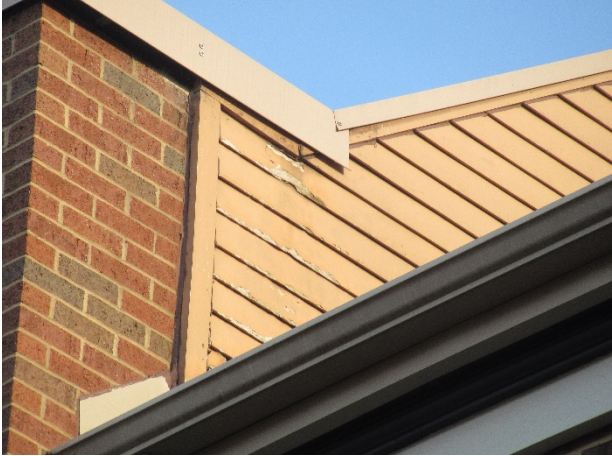
Parapet wall finish deterioration
