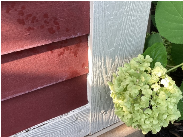
Lacking sealant at Unit 45
