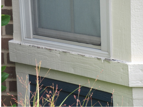
Finish rot and deterioration
