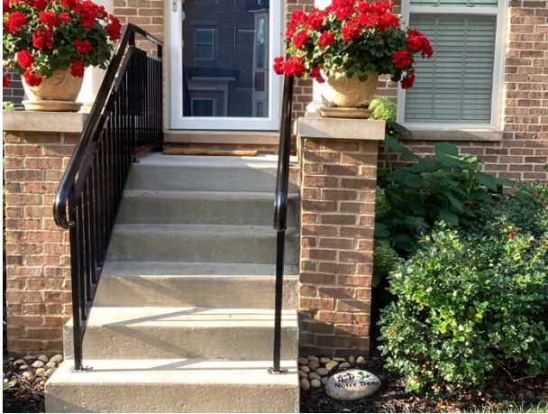
Leaning railing at Unit 67
