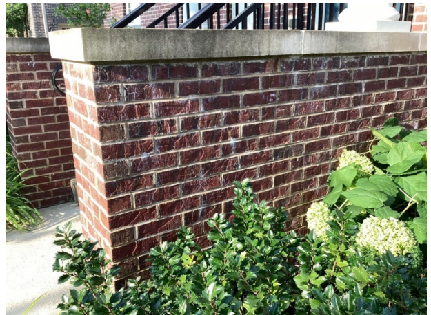
Wing wall efflorescence at Unit 71
