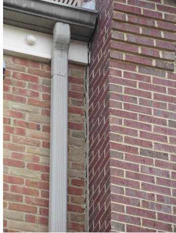
Brittle sealants and cohesive failure at Unit 72
