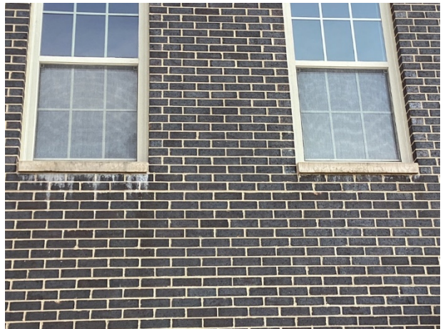
Efflorescence and sill cracks at Unit 92
