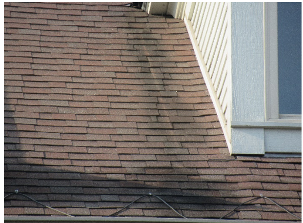
Asphalt shingle roof staining
