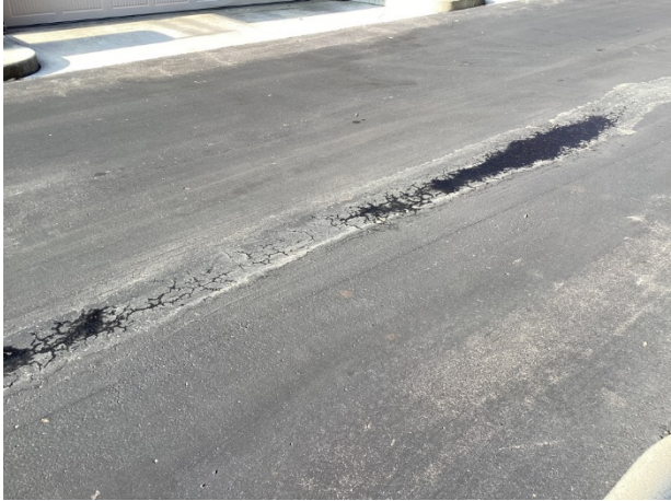
Standing water and cracks
