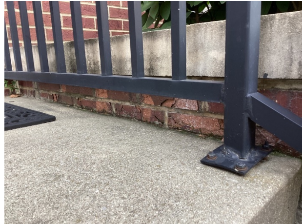
Spalled masonry at 1246 Duey Street
