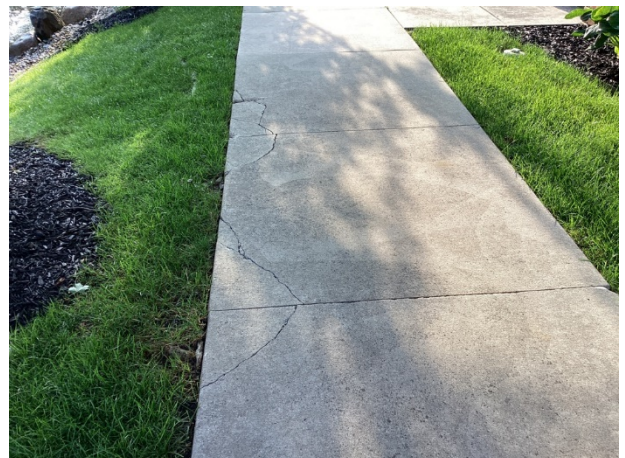
Sidewalk edge cracks likely due to settlement
