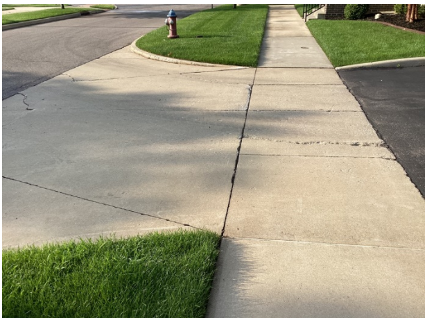
Cracks and spalls at concrete apron
