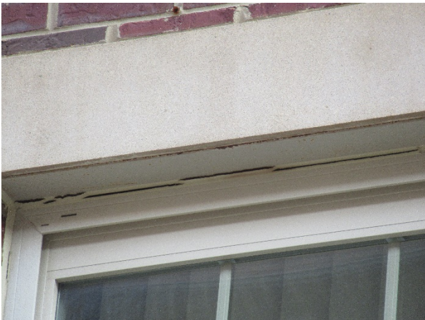
Sealant failure at window at Unit 72
