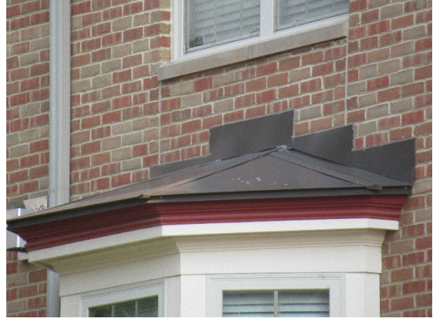
Metal roof with minor finish deterioration
