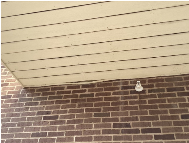
Soffit displacement at the unit owned balcony
