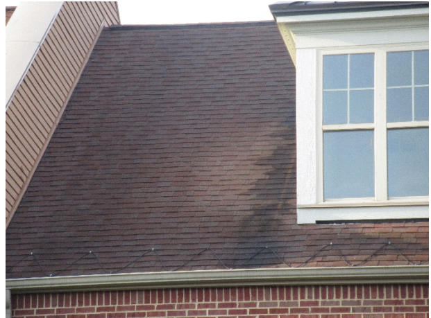
Asphalt shingle roof staining
