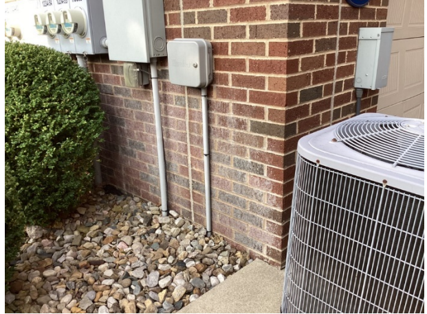
Efflorescence at Unit 55
