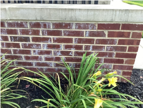
Efflorescence and masonry cracks at Unit 24
