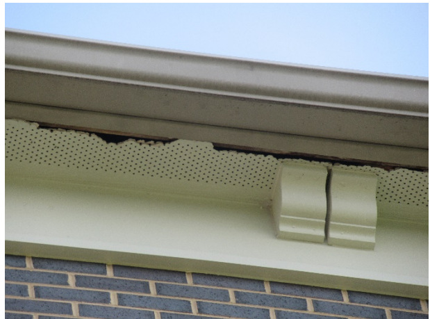
Missing soffit at Unit 98
