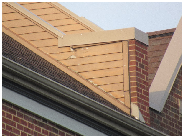
Parapet wall finish deterioration
